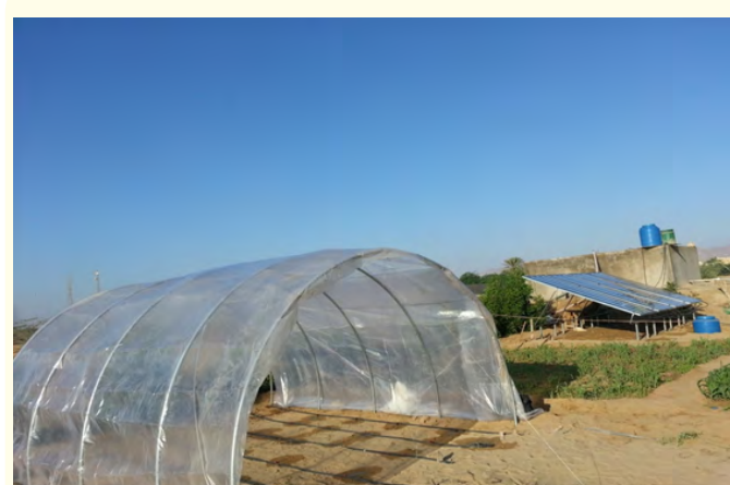
Figure 6: Solar desalination and Drip in tunnel at Gadani Hub, Balochistan.
