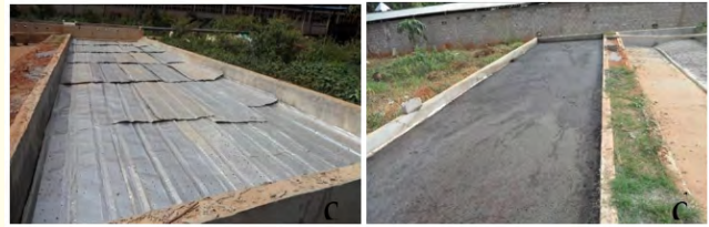
Figure 10: Construction of the drying bed (a- Placement of the drain; b- Placement of the gravel pack; c- Bed ready to receive the slurry; d- Bed loaded with slurry).
