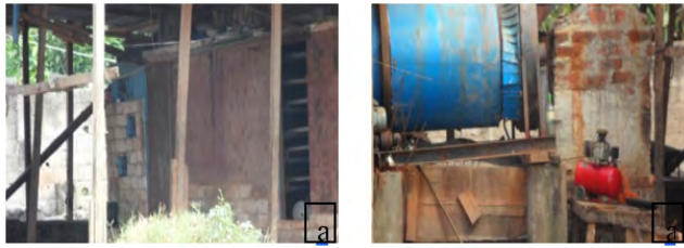
Figure 7: Defective drying equipment (a- Paddle oven; b- Rotary cylinder).
