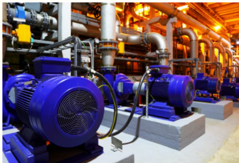
Figure 5: The utilization of large motors inside different stations.
